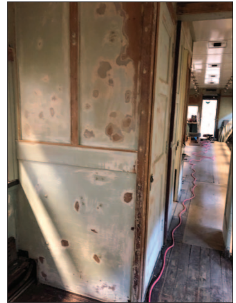
▲ The interior of the car had been prepared for painting in this photo, taken in mid-July of 2020.
