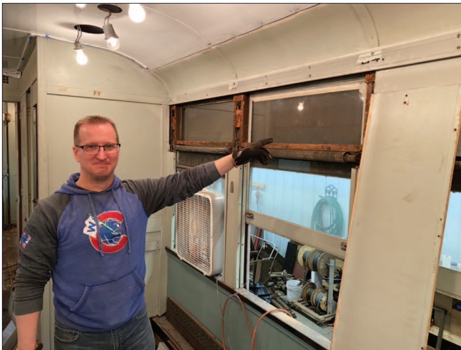
▲ Eric Zabelny points to an open window after it had been cleaned and repaired so that it would open properly. Rotten wood and window frames were repaired or replaced, ensuring that this restoration was more than cosmetic. Eric is another former volunteer who rejoined the railroad to help with Car 761, a restoration project he worked on the first time it started.—Tom Fleming photo
