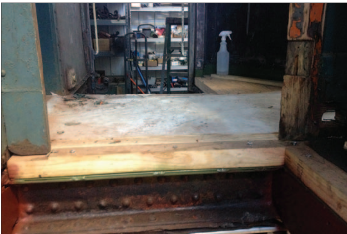
▲ Wood sub-flooring and trim were installed in the east end vestibule by late May of 2020.
